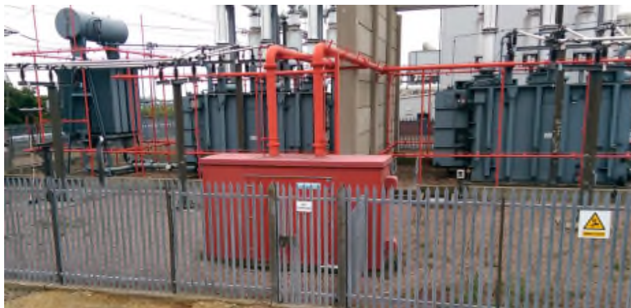
Figure 2.5.7: Transformer Automatic Foam System
